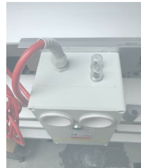
JB 176-00-180 supporting a transformer
