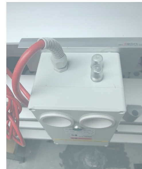
JB 176-00-180 supporting a transformer
